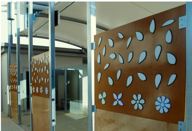
Playground Panels - external view during installation. The pattern motif unifies the artworks
